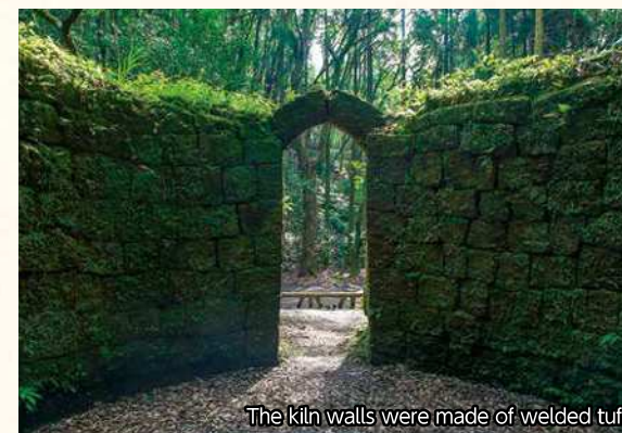
The kiln walls were made of welded tuff *The area surrounding the Terayama Charcoal Kiln is off limits due to disaster recovery work.
